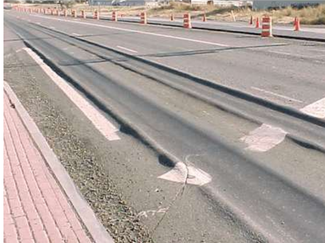
Figure 2.13 Rutting in asphalt pavement [127].
