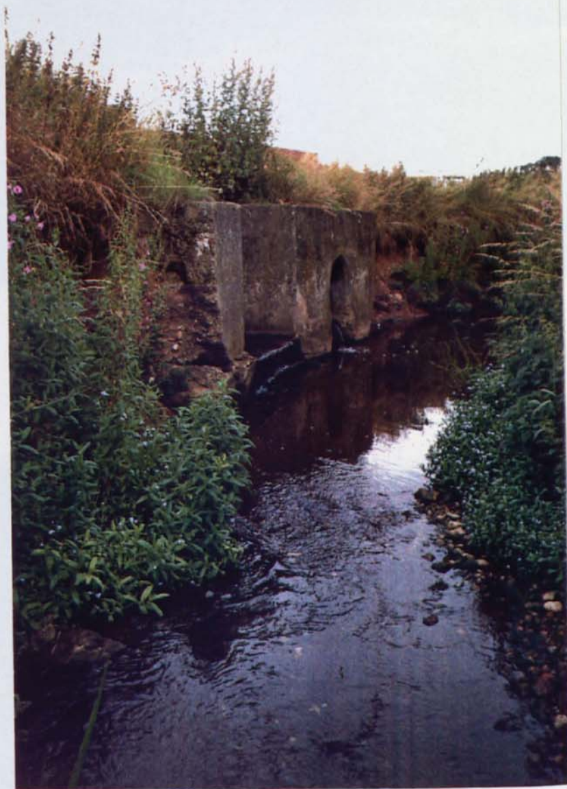
(x) Site 28 Twin outfalls to Whetstone Brook, Leics. from an industrial estate and M1 motorway
