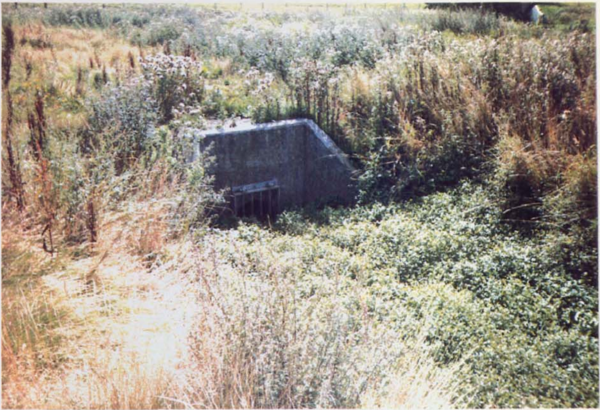
(iii) Site 15 Weed growth at outfall from airport
