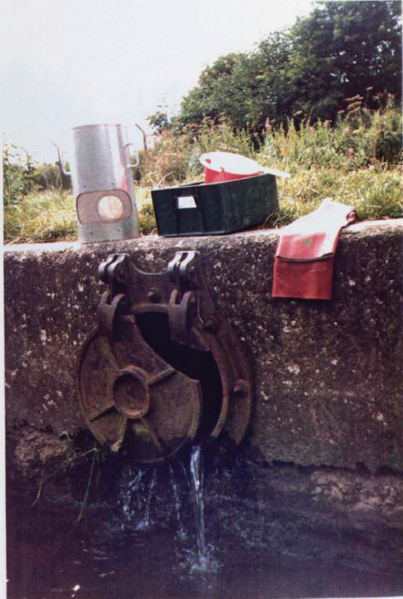
(ix) Site 31 Outfall to R. Blithe, Staffs., showing dry weather sewage flow
