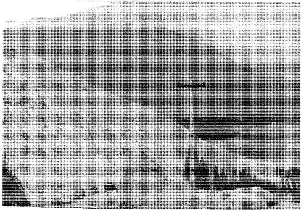
Plate 1.7 Unstable slope at km 56. Shangoldeh is located at the bottom right hand corner of the picture.
