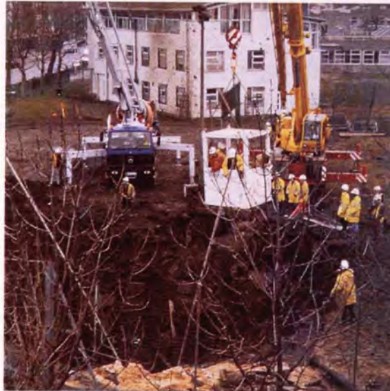
Figure 3.5 – Engineers examining site of blow-out DLR contract (NCE, 2004)
